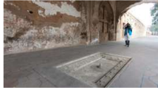
Figure 44: Fountain's condition after restoration at interior of north gate, original openings at right have been bricked over.
