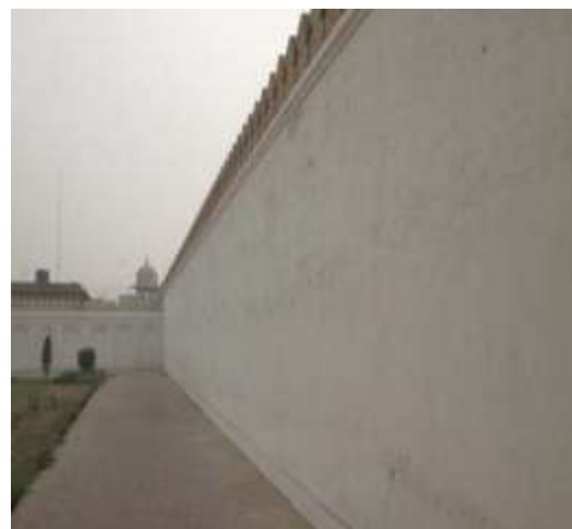
Figure 40: After Conservation "Protection work of Lime Plaster of Perimeter wall of Naqqar Khana"
