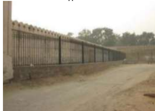
Figure 38: After Conservation "Plinth Protection and Fixing of iron grill on exterior side of perimeter wall of Naqqar Khana"
