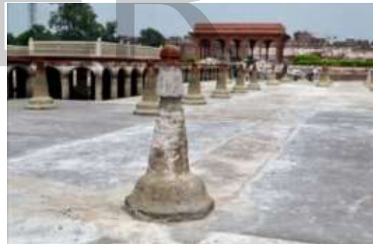
Figure 50: Deteriorated condition of fountains
