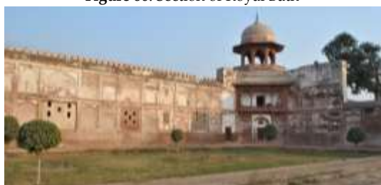
Figure 81: The Royal Bath stretches south(left) from the tower. Note the three sets of windows set into the bath wall
