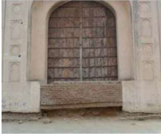
Figure 41: Condition before Restoration of wooden north gate at Naqqar Khana Complex
