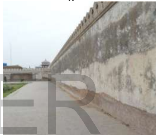
Figure 39: Before Conservation "Protection work of Lime Plaster of Perimeter wall of Naqqar Khana"
